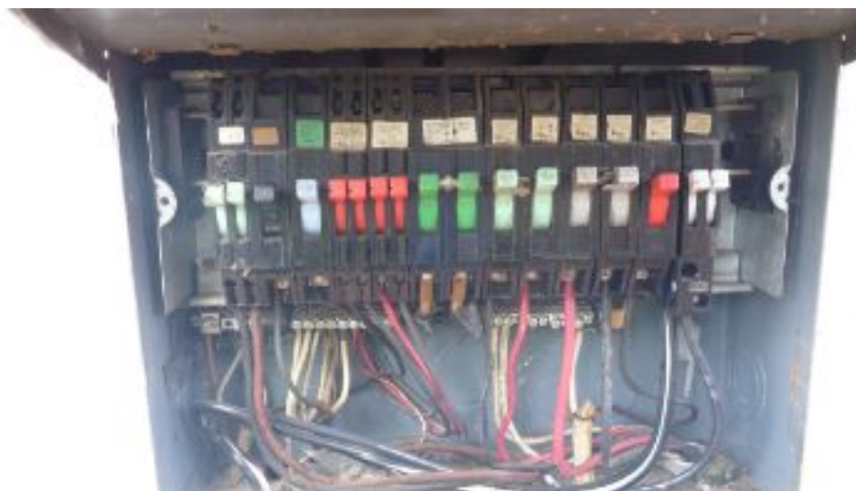
Panel needs an interior cover
