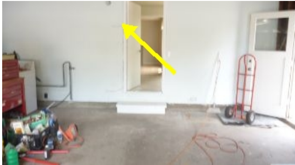
Door going into house needs self closing hinges
