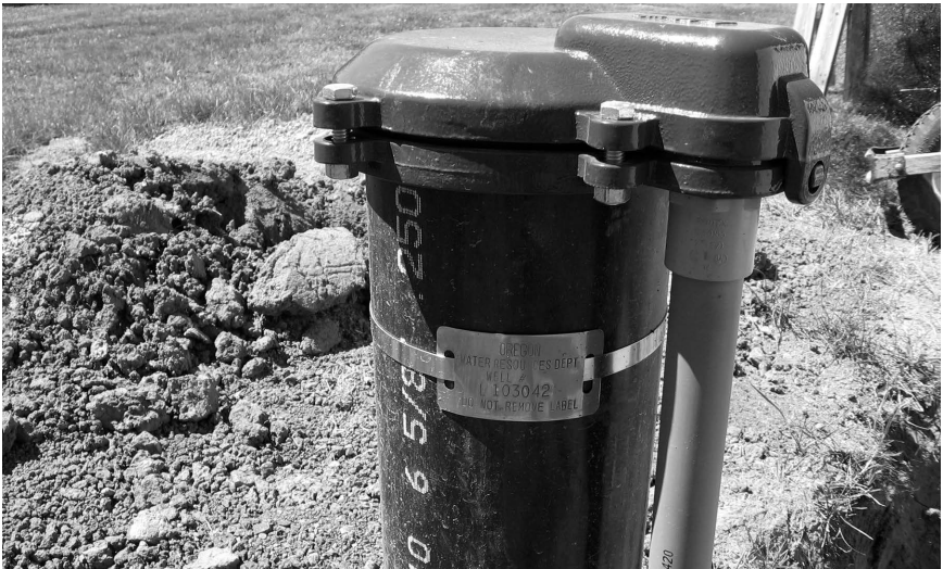
A metal well label, displaying the well ID number, should be on every well.
